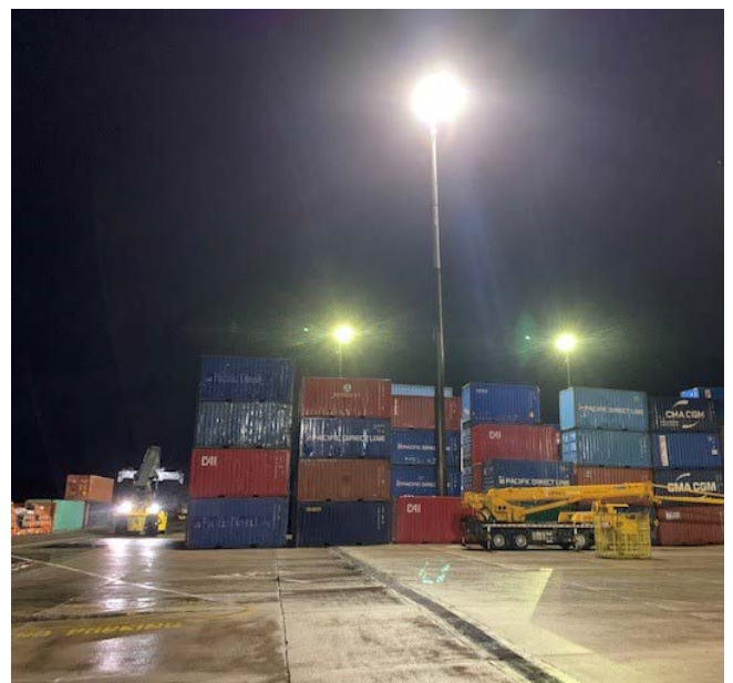
Upgraded tower light with smart LED lighting at Port of Suva.
